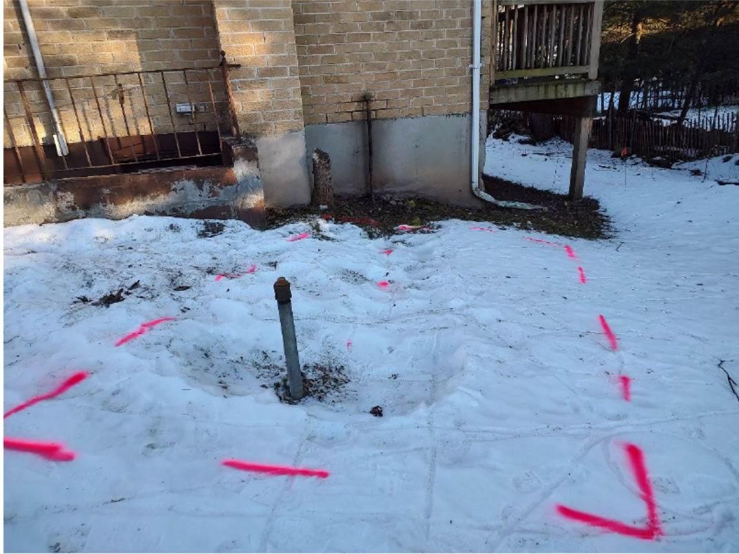
Photo 3– View of the UST providing fuel oil to Building #4.
